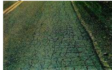
Fig. 1: Bad fatigue cracking.
